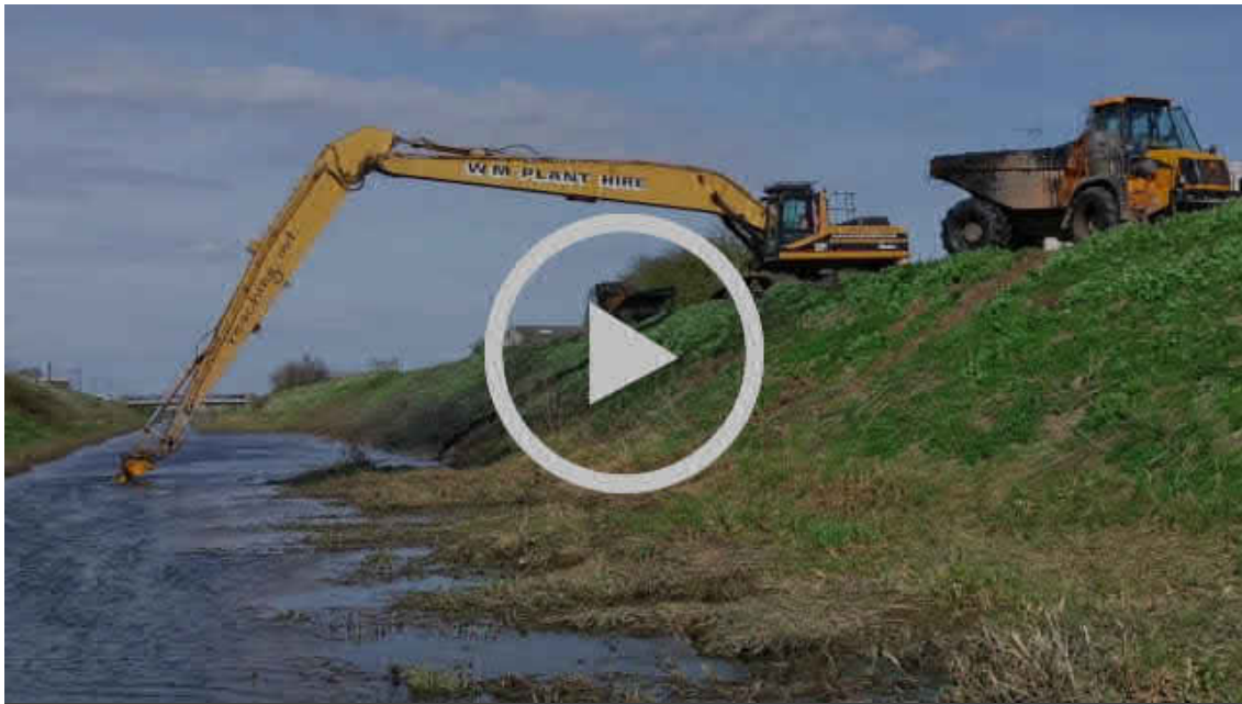
Working with Black Sluice IDB on weed clearance in the South Forty Foot Drain mitigating future flood risk.
